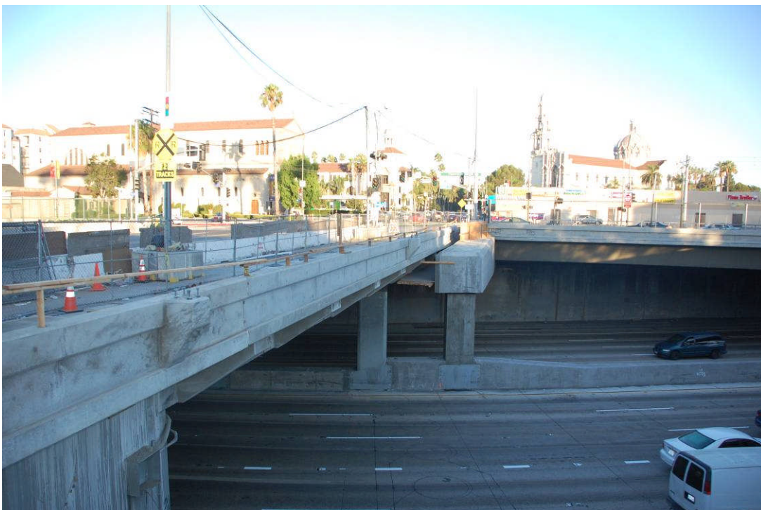
Looking at the exterior of the widened Adams bridge from the top of the POC looking west.
