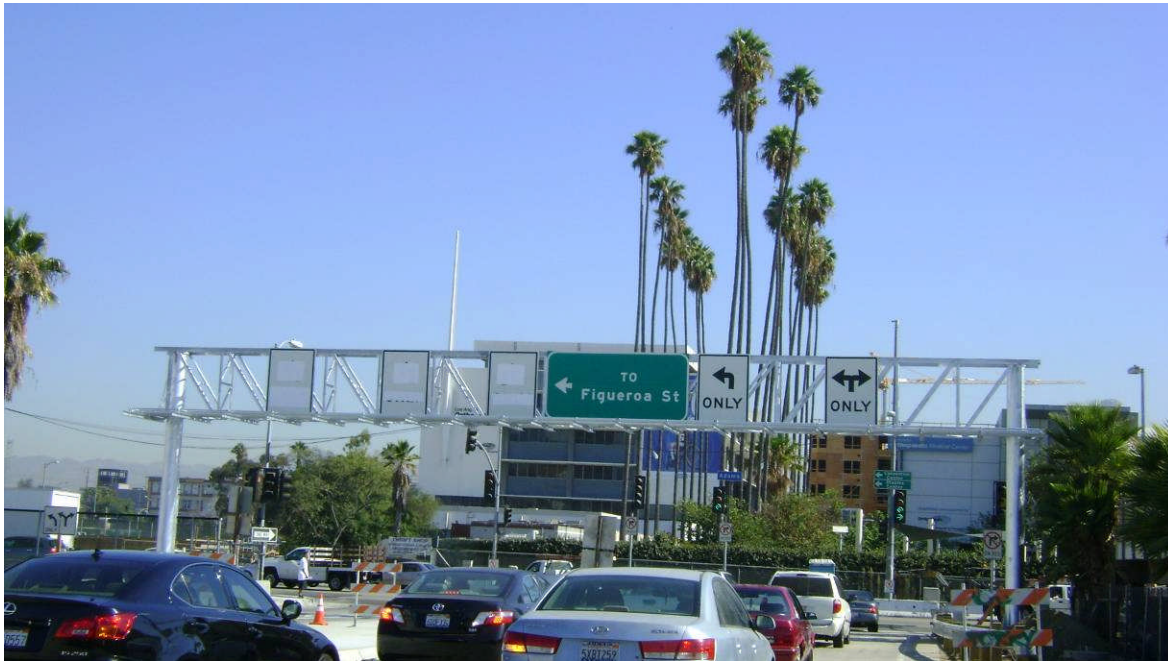
New sign at Adams looking North from bottom of newly poured ramp.
