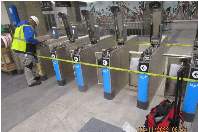
Programming and software testing of fare gates at MLK Jr Station
