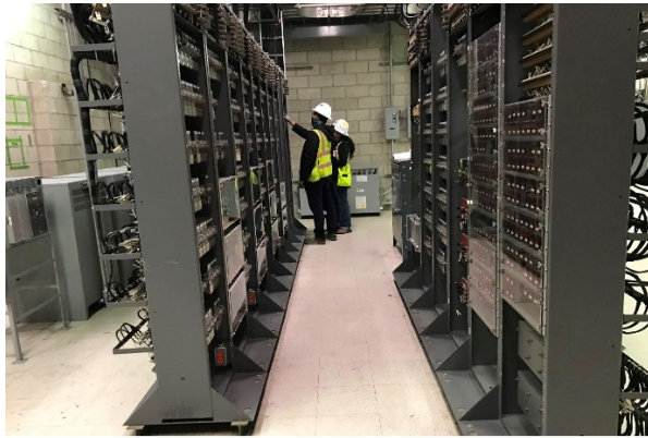
Inside TCC Room at Wilshire/Western Station
