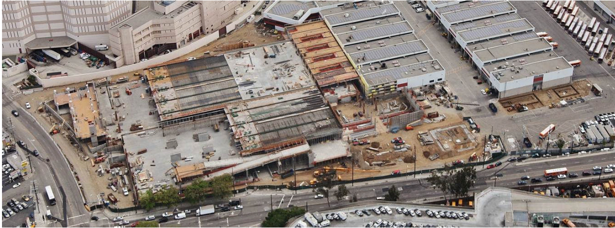
April 2014 Transportation Building, Parking Garage and Maintenance Building in construction; at the bottom side Cesar Chavez Avenue and at the left side Vignes Street.
