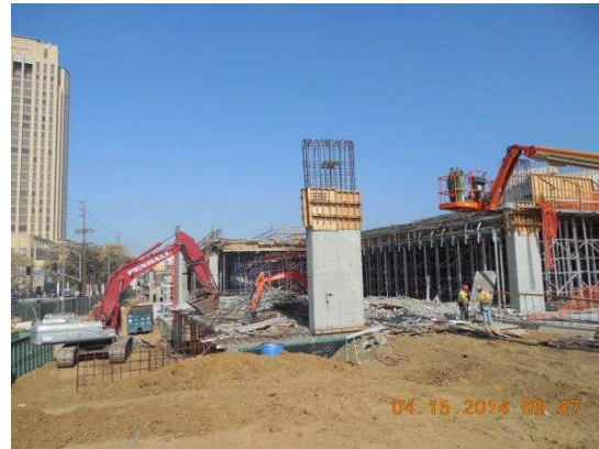
1 st phase surgical demo collapsed upper Deck #14 debris.
