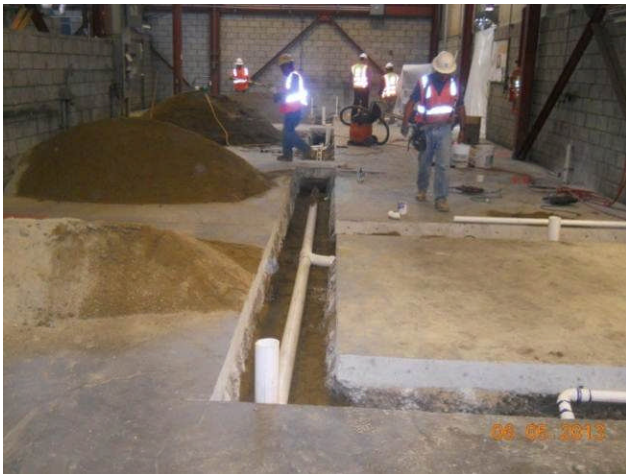
Radiator shop plumbing work.
