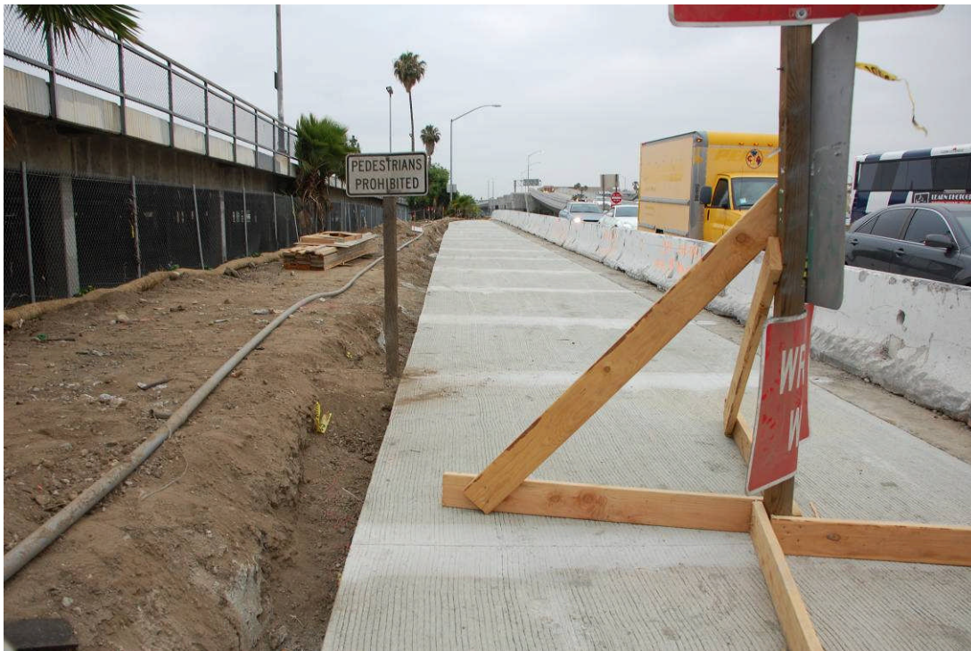
PCCP at Adams off ramp.
