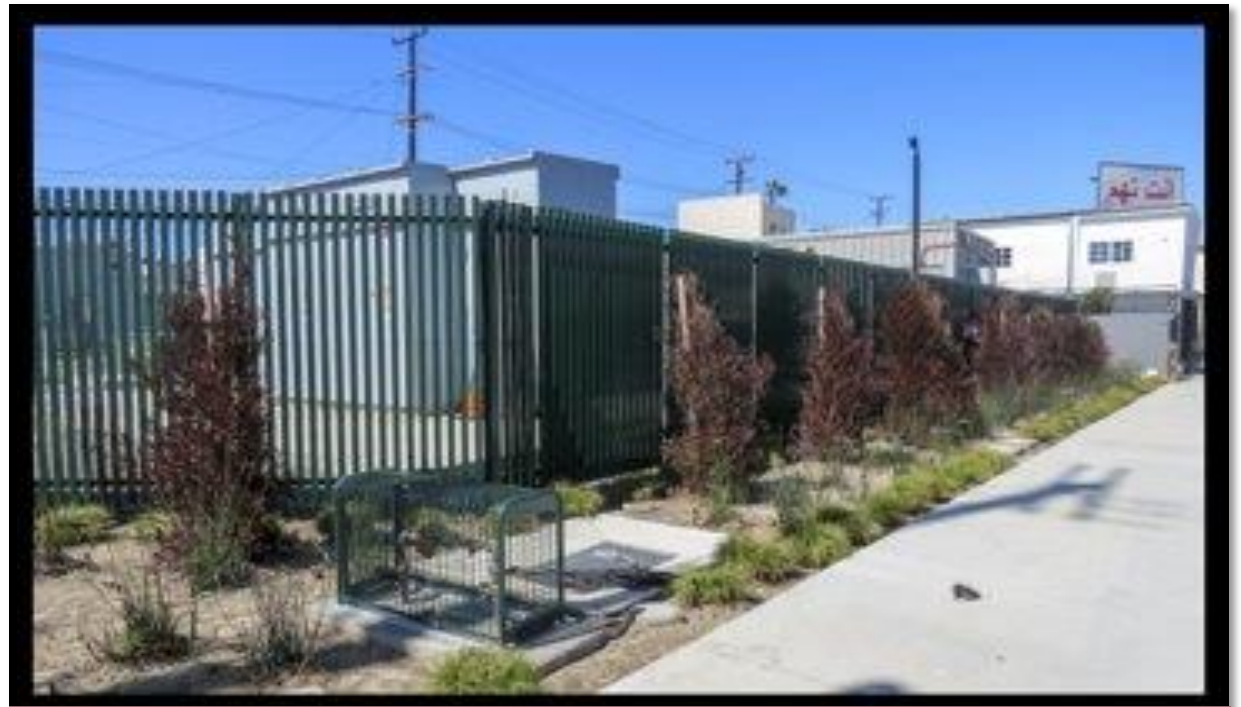
Metro K Line TPSS in Park Mesa Heights
