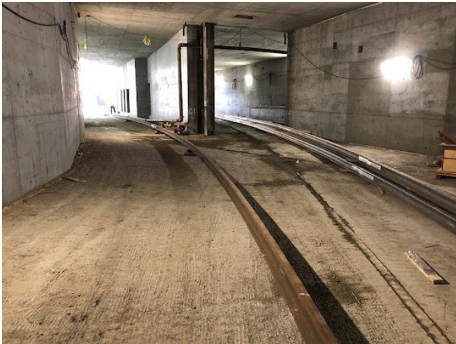
400' CWR stringers being pulled into right tunnel on rollers at 1st St Leg
