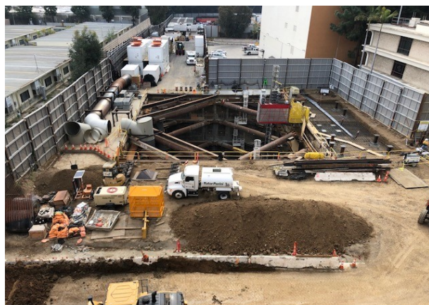
Access Shaft in Century City
