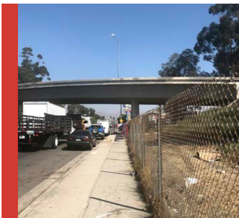
Inadequate sidewalk, no buffer from heavy traffic for pedestrians, no shade
