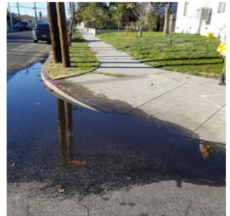
Drainage issues at intersection make access ramp hard to use
