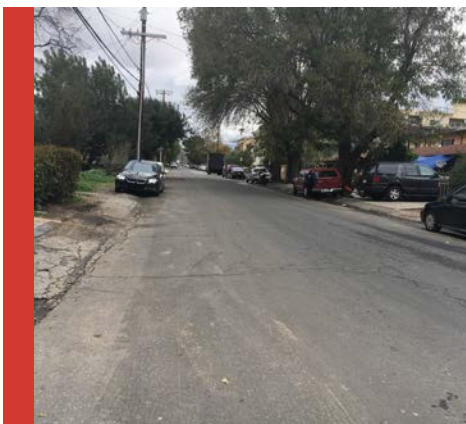
Missing sidewalks on Cedros Ave north of Vanowen St
