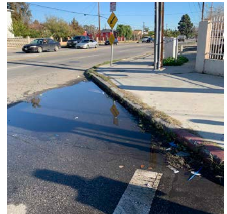
Missing ADA access ramps and drainage issue reduces accessibility
