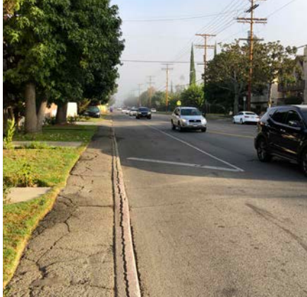
Uneven asphalt sidewalk with no raised curb
