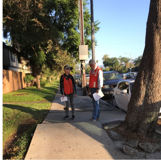
Technical team members encountering sidewalk vertical uplift near Woodman Station
