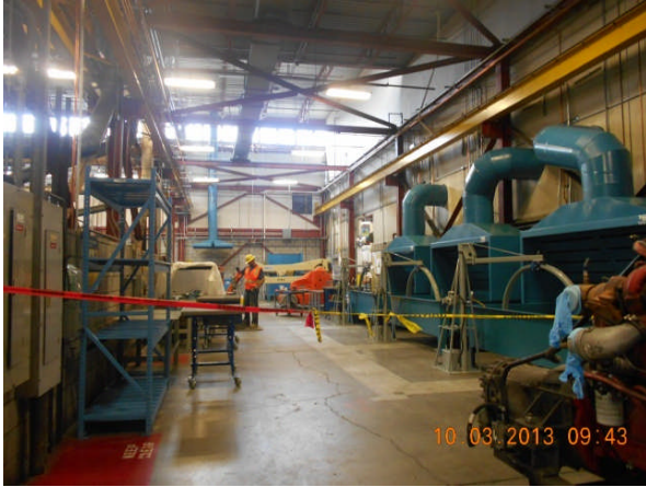
Exhaust fan ducts and radiator lift arcs at Radiator Shop.
