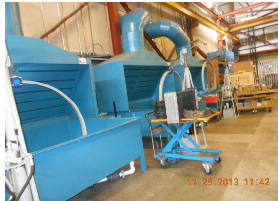
Radiator Shop leak tank detectors and lift equipment.
