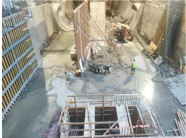
Interior wall preparation at the east end Track Level at Historic Broadway Station
