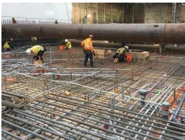
Bottom mat rebar installation at Upper Ancillary at Grand Av Arts/Bunker Hill Station
