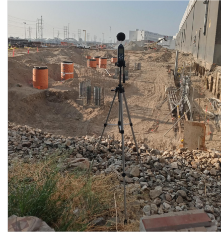
Sound monitoring equipment.
