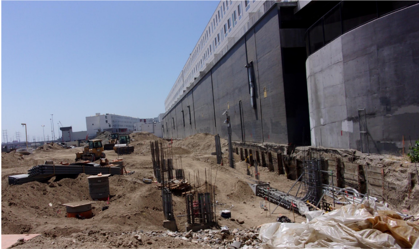
Looking south at the new TPSS where conduits and manholes have been installed.
