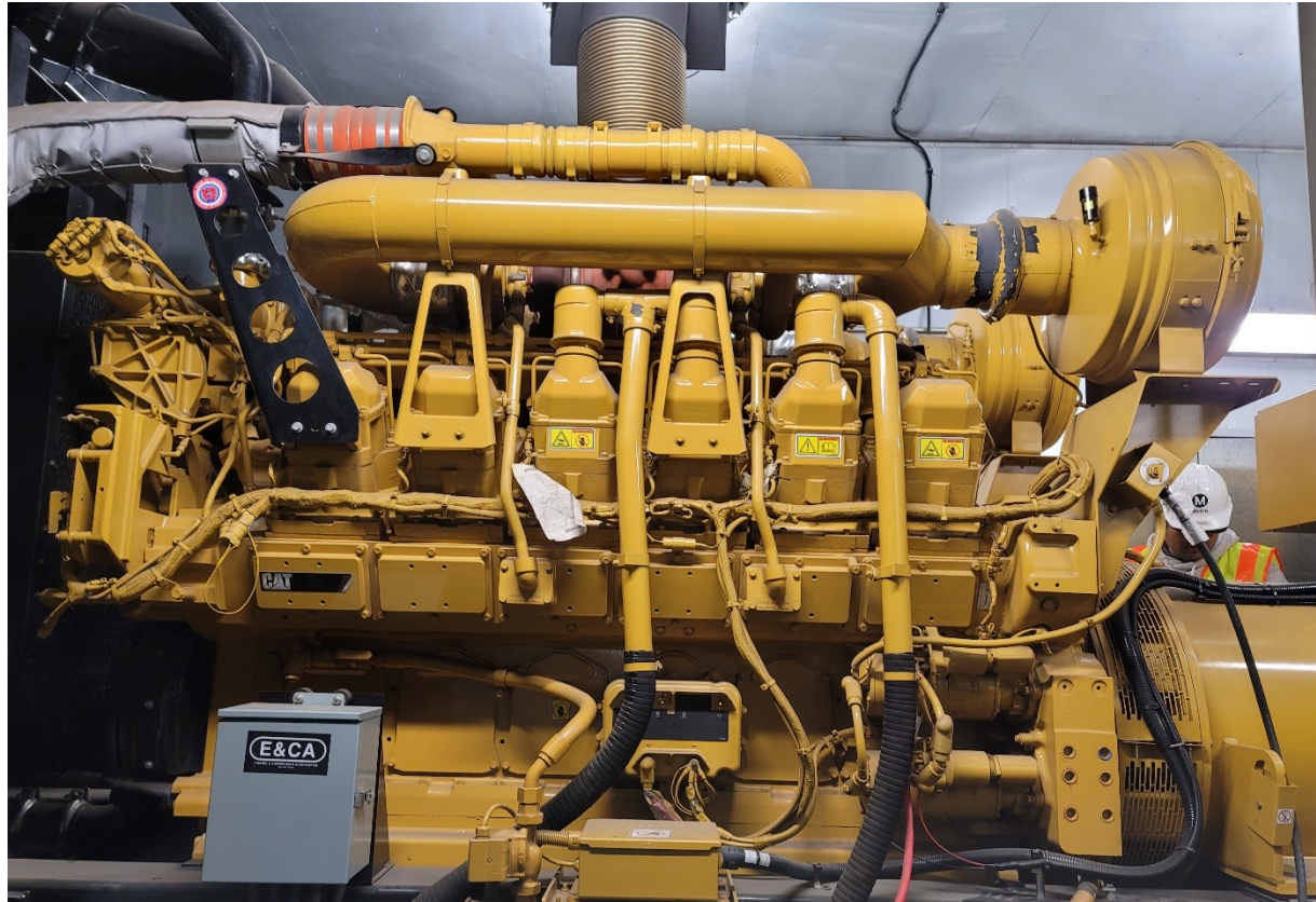
EBPS Generator Live Load Testing
