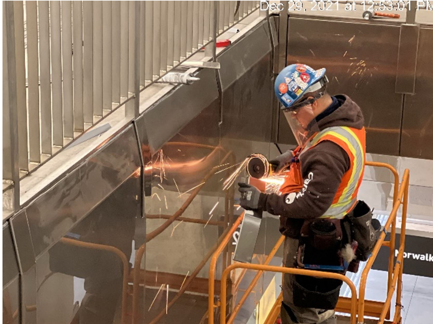
Installing stainless-steel cladding trim plates to the interior guardrail posts around the perimeter of escalator
