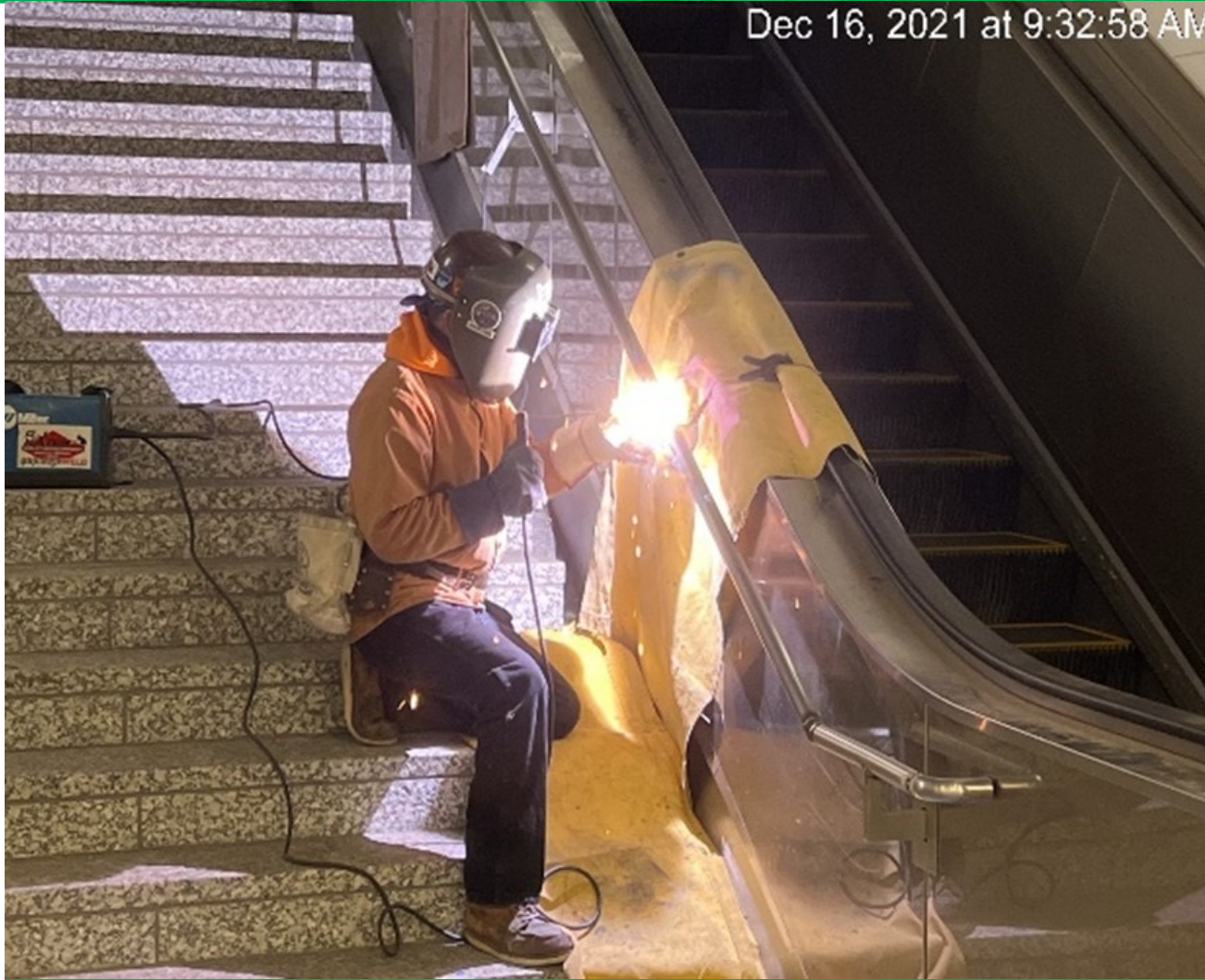
Installing handrails along the exterior sides of escalators between the intermediate landing and concourse
