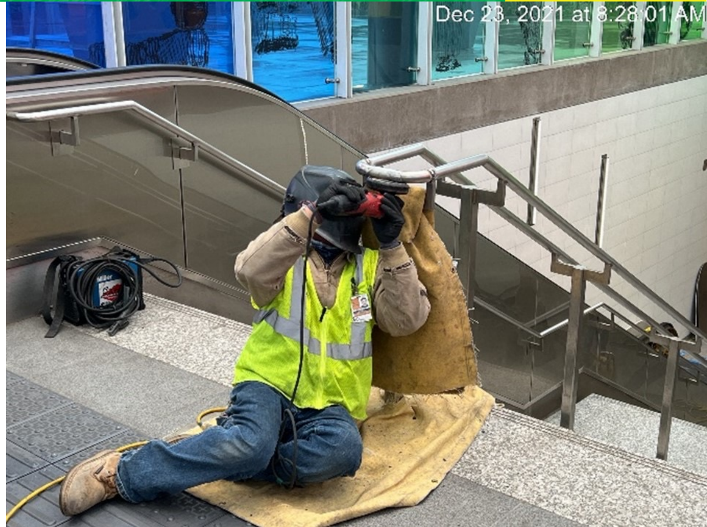
Welding handrail return to staircase at the main entrance of the Leimert Park Station
