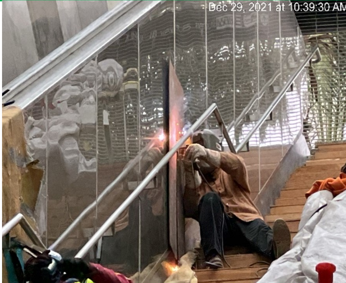
Welding handrails along the exterior sides of the escalators at the main entrance
