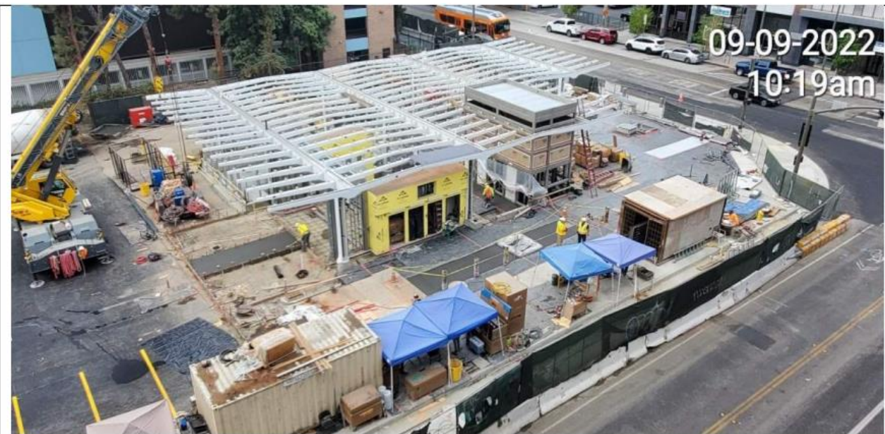
Placement of architectural concrete paving at the east section of Broadway Plaza
