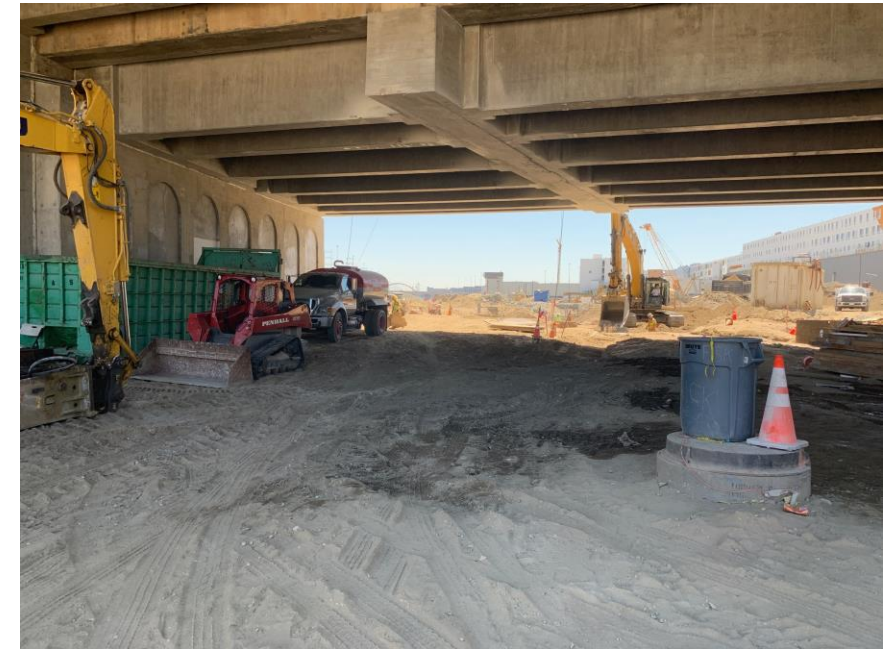
Bent removal complete. Overhead girders were joined to support the bridge before of Bent 16.
