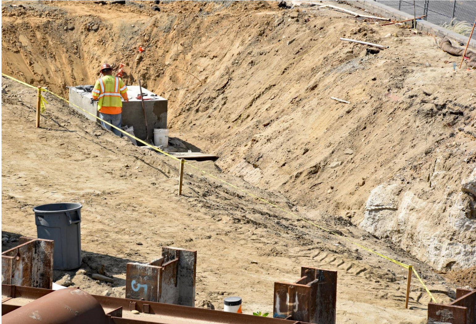
Workers continue installing the storm drain along Center St near Commercial St.
