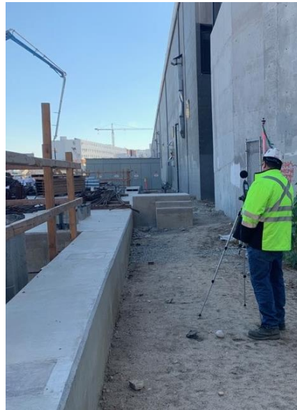
Noise monitoring equipment near One Santa Fe.
