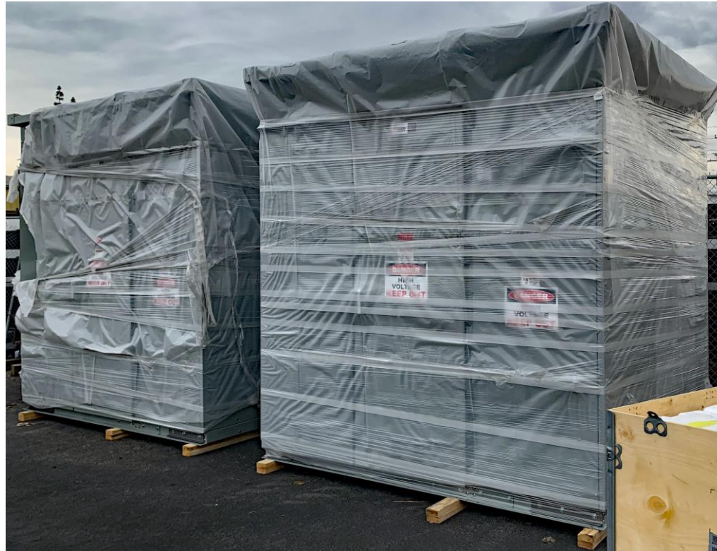
Power cabinets when they arrive on site.
