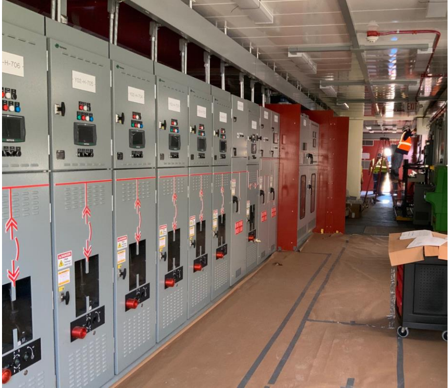
Inside a typical Traction Power Substation.
