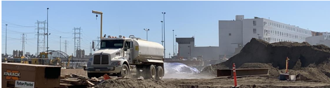
Watering truck can be seen in the background east of the One Santa Fe building.
