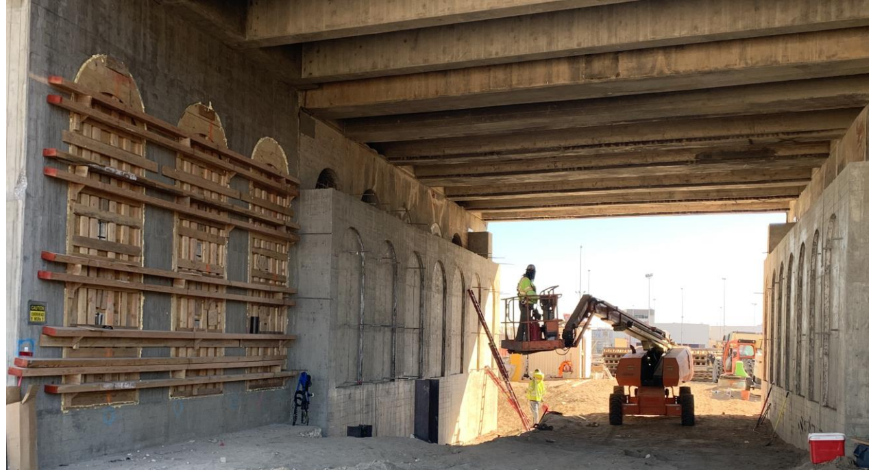
Completed support in preparation for girder installation under the 1st Street Bridge and infill of walls.
