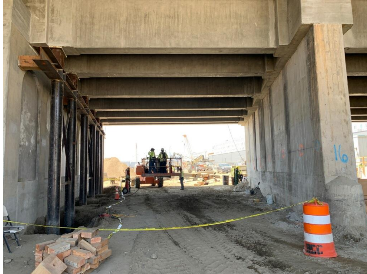
Concrete infill have been completed for bents 15 and 16. All falsework here has been removed.
