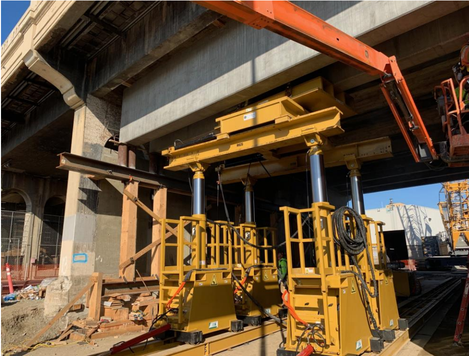
Installation of a edge girder underneath the 1st Street Bridge in the Arts District
