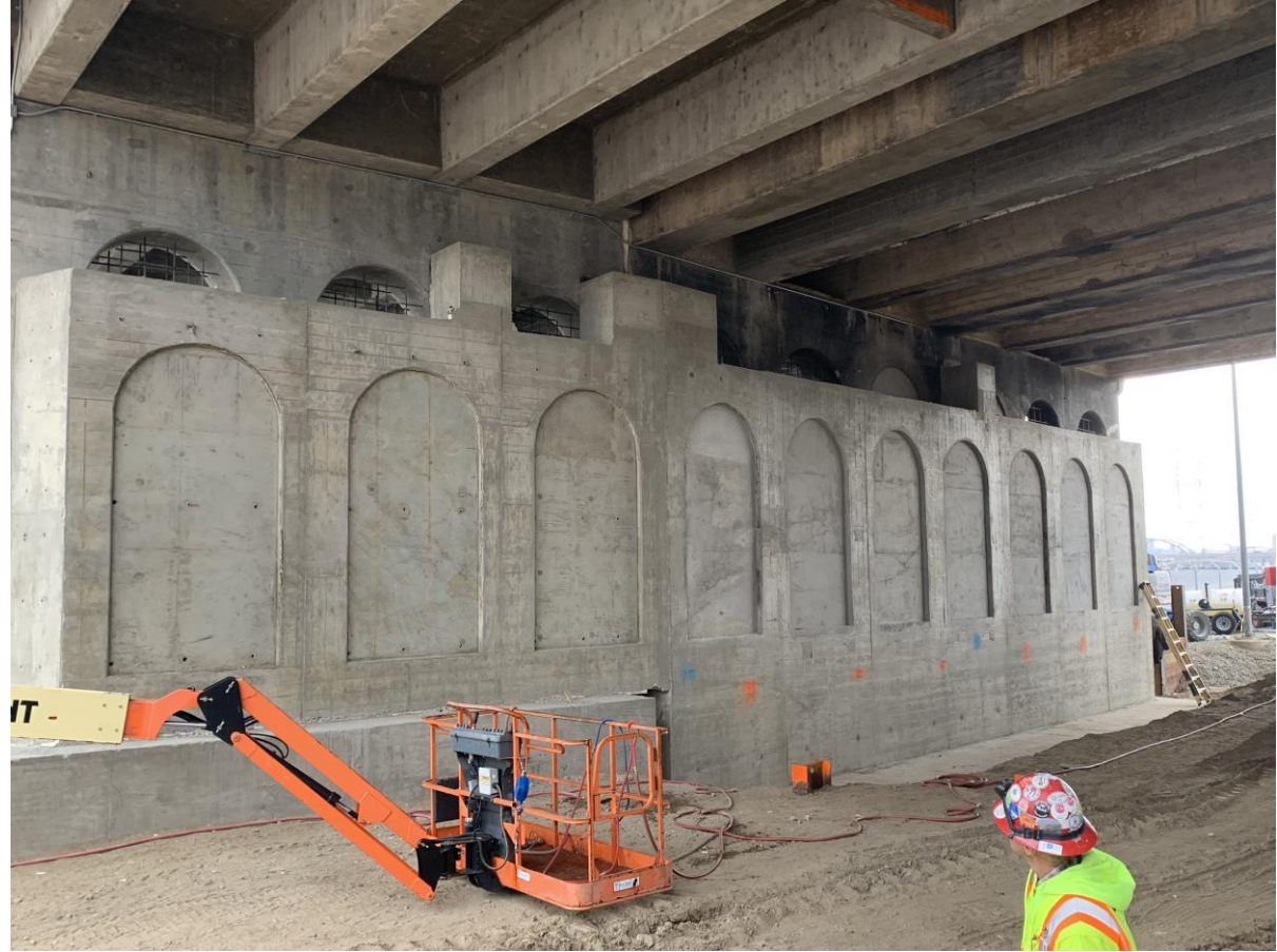
Completed structural wall prior to installation of girders and the demolition of selective support bents.
