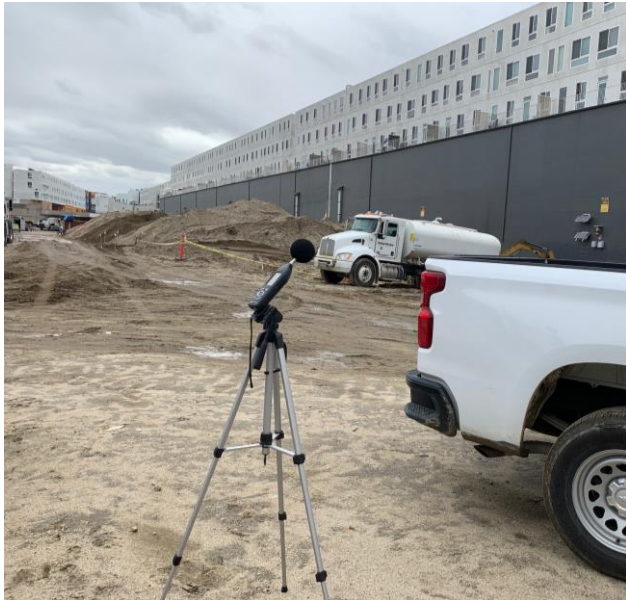
Watering truck can be seen in the background immediately east of the One Santa Fe building.
