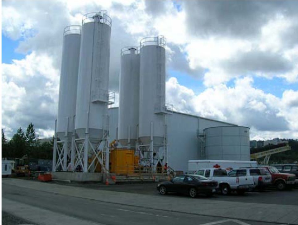
Figure 4-13. Enclosure with Materials Storage Silos, Eastside CSO Project, Portland, OR
