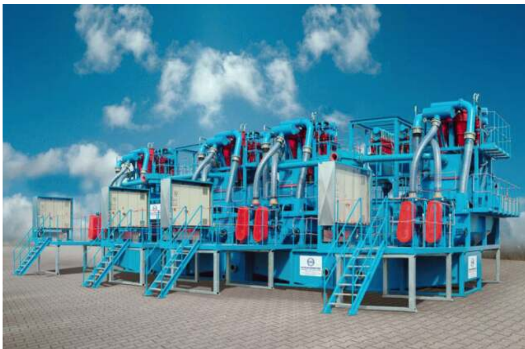
Figure 4-12. Slurry Treatment Plant, Westside CSO Project, Portland, OR
