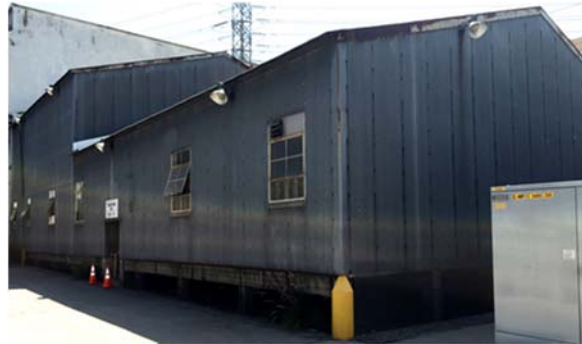
Building 11A: Transformer Test Building, 1961, (19-176372). Camera facing NE. Photo ICF International, July, 2016. IMG_9118.jpg
