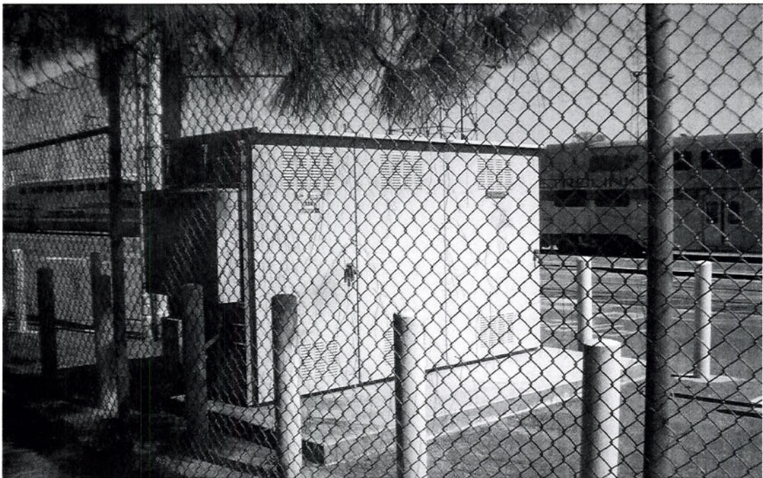
Photo 8 Electrical panel, near entrance
