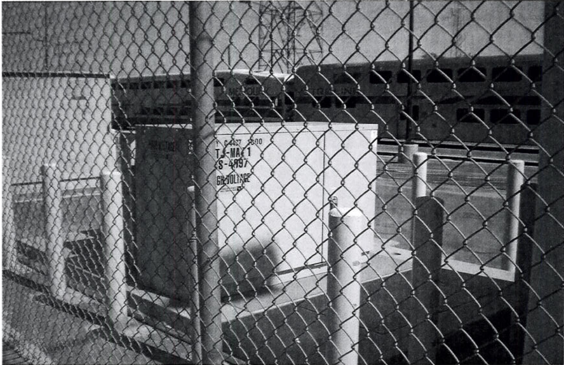
Photo 7 High voltage transformer, near entrance
