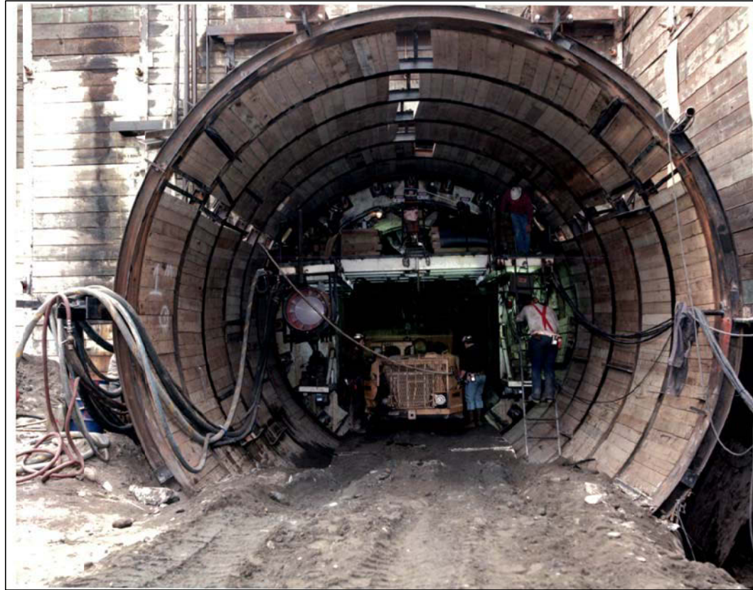
Photo No. 1. False tunnel sets at the South Tunnel Portal of YR Tunnel (south of LAUS) with tunnel shield and mucking machine in the background. Photo taken: 01/30/90. Source: SCRTRD, 1990a.
