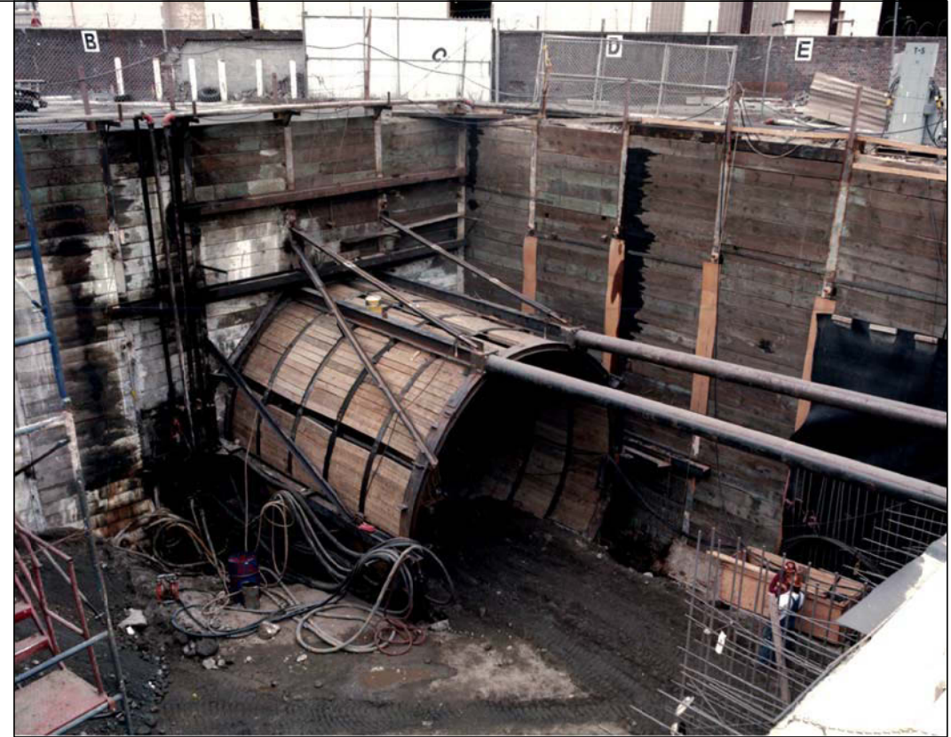
Photo No. 2. False tunnel sets and the jacking frame and struts for pushing the shield off of at the South Tunnel Portal (south of LAUS). Photo taken: 01/30/90. Source: SCRTRD, 1990a.
