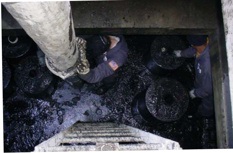
Pollutants must be removed to restore the StormFilter to its full efficiency and effectiveness.
