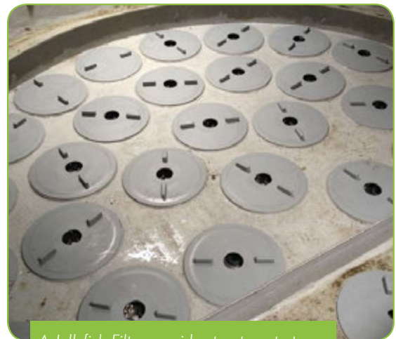
A Jellyfish Filter provides treatment at an Industrial Park in Lake Tahoe, Nevada.
