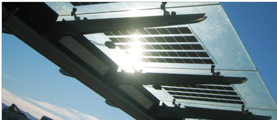
◀ Solar paneled canopies protect from the sun while harnessing its energy to power the platform.
