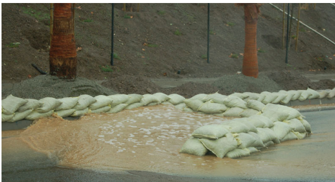
Controlling stormwater runoff during construction is critical to maintaining water quality in the Study Area.
