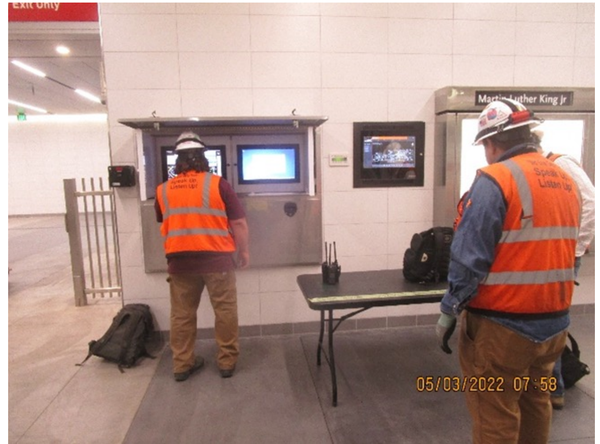
Scenario testing for the emergency ventilation fan flow switch sensors
