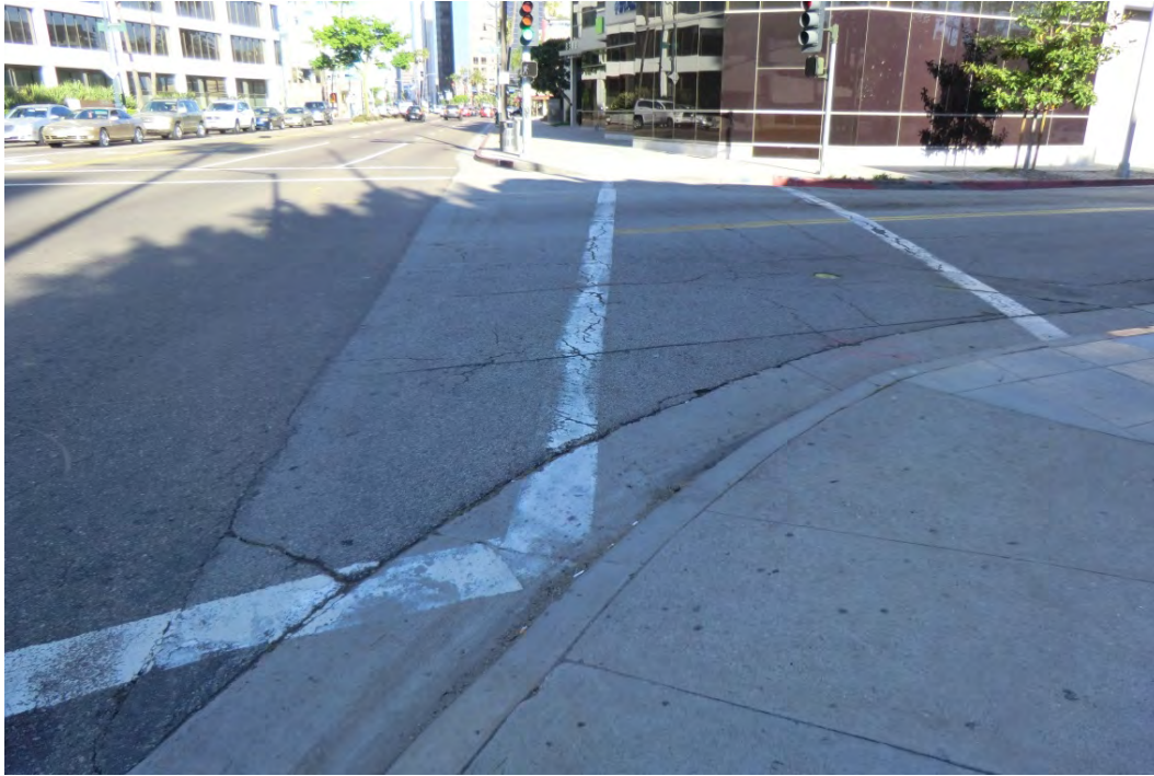
Figure 2-1: Inadequate Clear Zone
