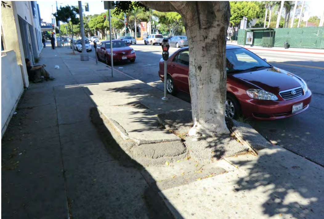
Figure 3-1: Sidewalk Uplift Caused by Ficus Roots
