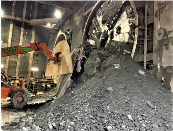
Twin tunnel boring machines (TBMs) being used on the D Line Subway Extension Project currently under construction.
