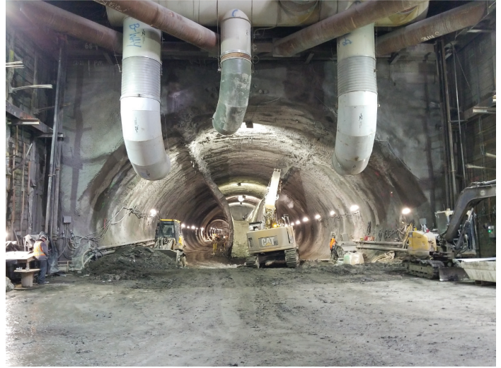
An image of Sequential Excavation Mining that was used to create a portion of the tunnel for the Metro A/E Lines in downtown LA.
