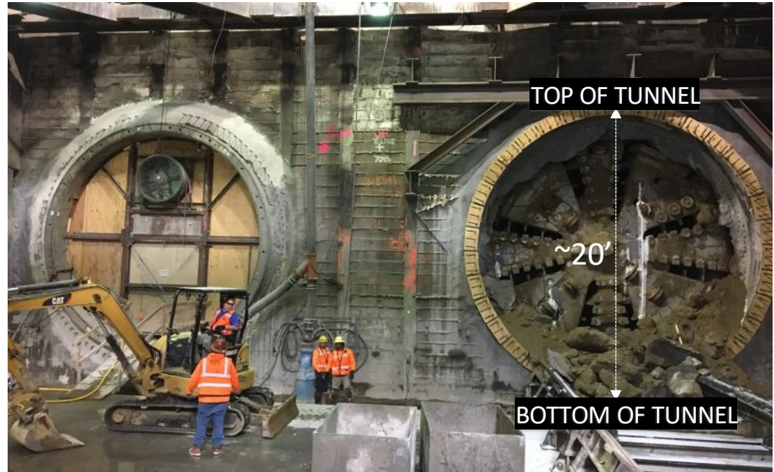
“Harriet” the tunnel boring machine at the K Line Leimert Park Station
