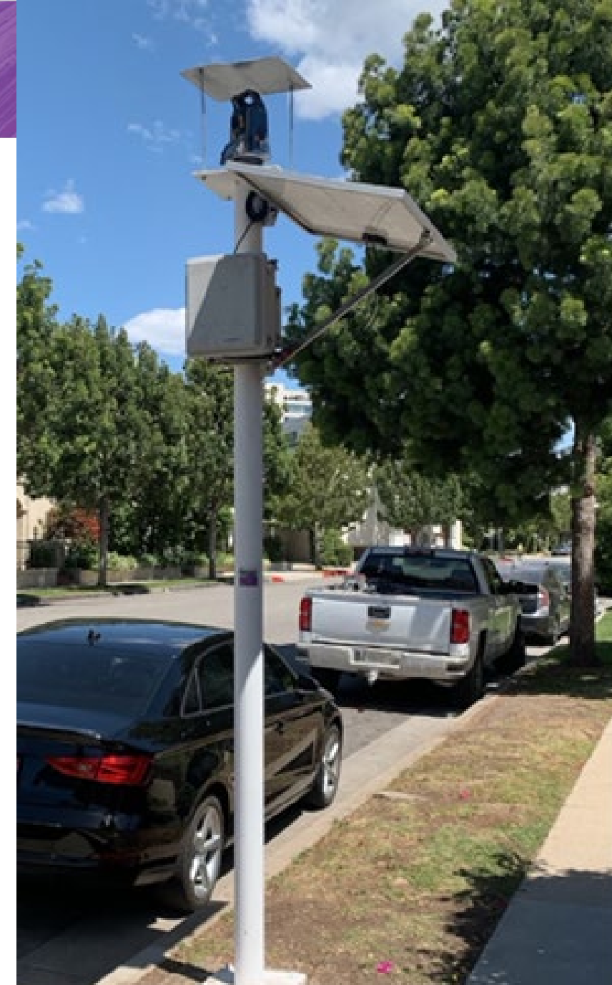
Example of 10-foot geotechnical instrumentation pole.
