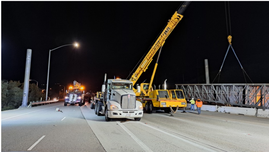
Crews preparing to remove existing overhead signage with crane and placing in center median
