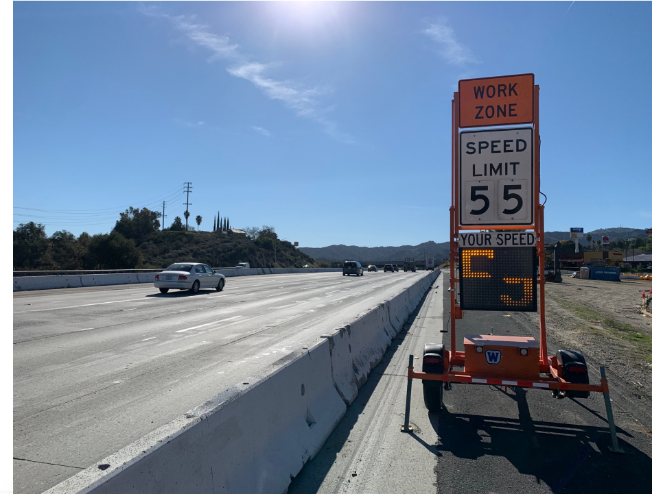
Work zone speed limit signage
