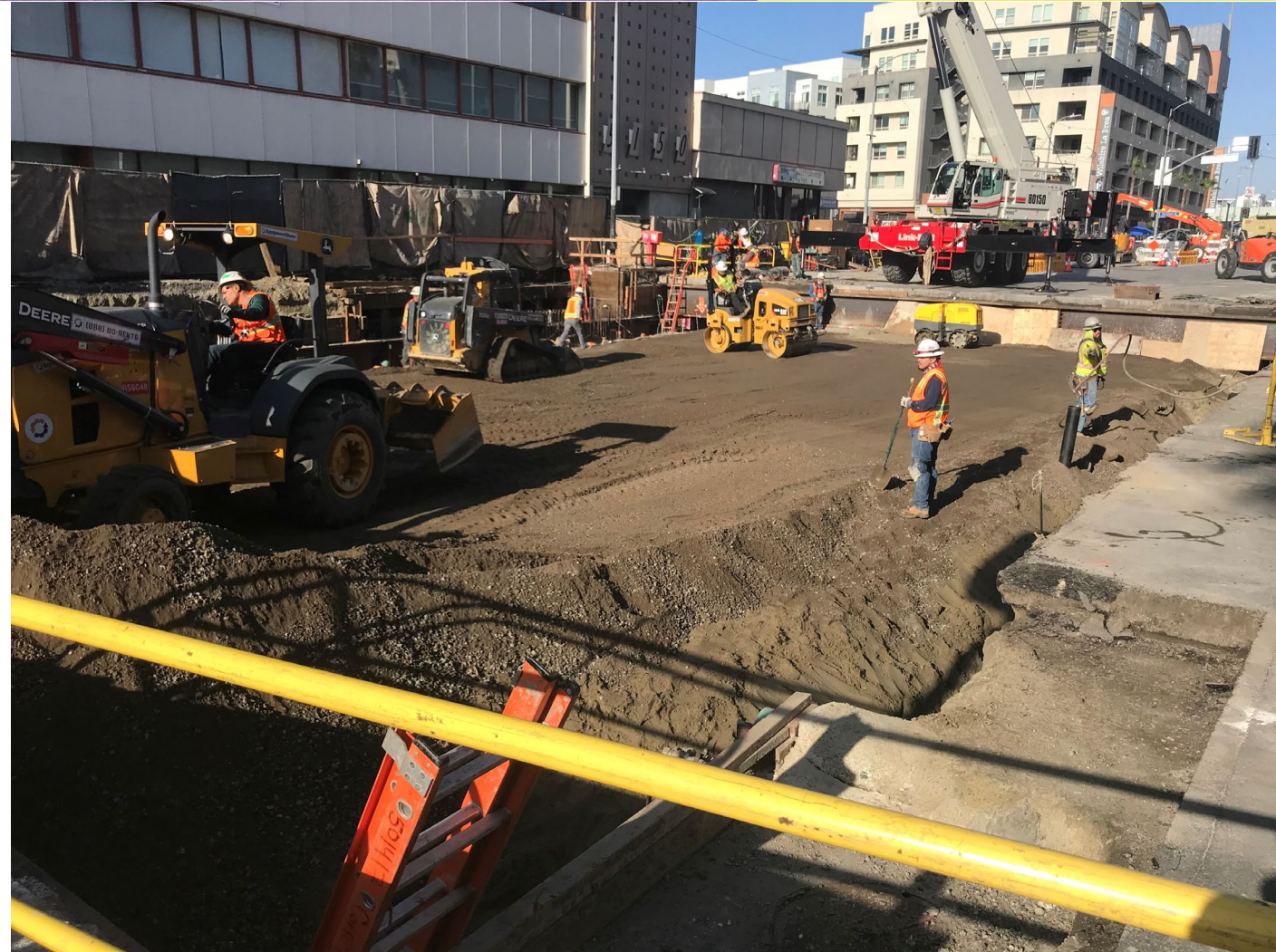
Backfilling operations at Wilshire Bl and Orange Dr, within the City of Los Angeles
