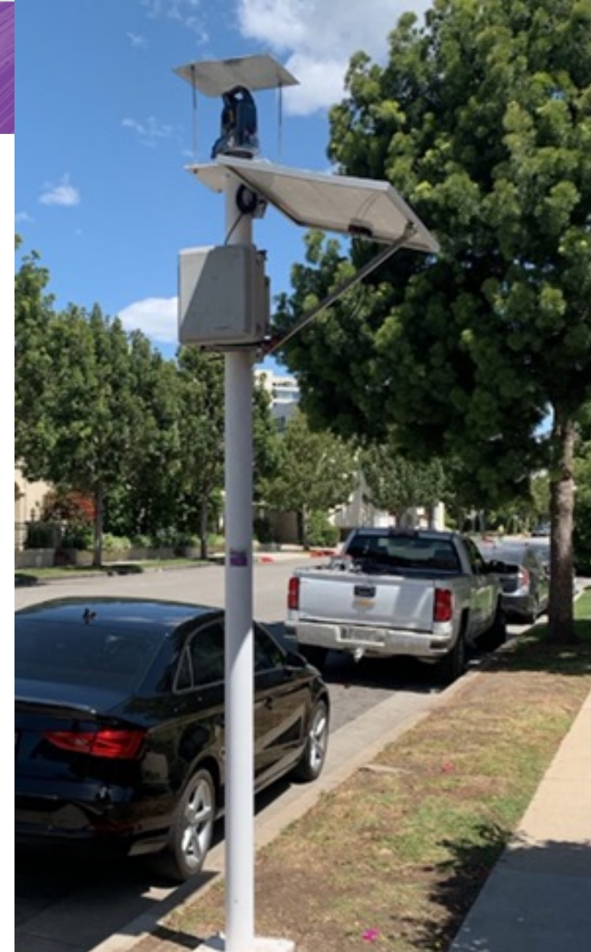
Example of 10-foot geotechnical instrumentation pole.
