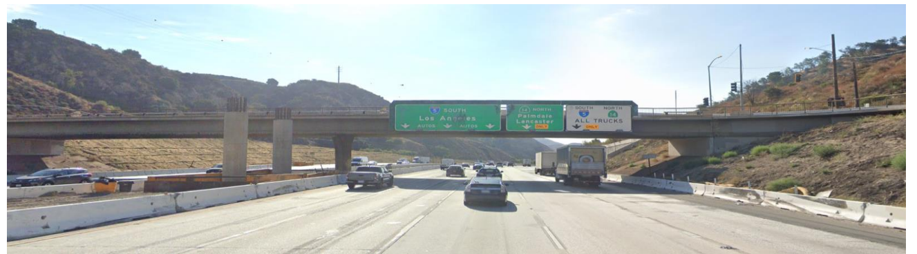
Existing sign structures that span the full width of the freeway that will be replaced
