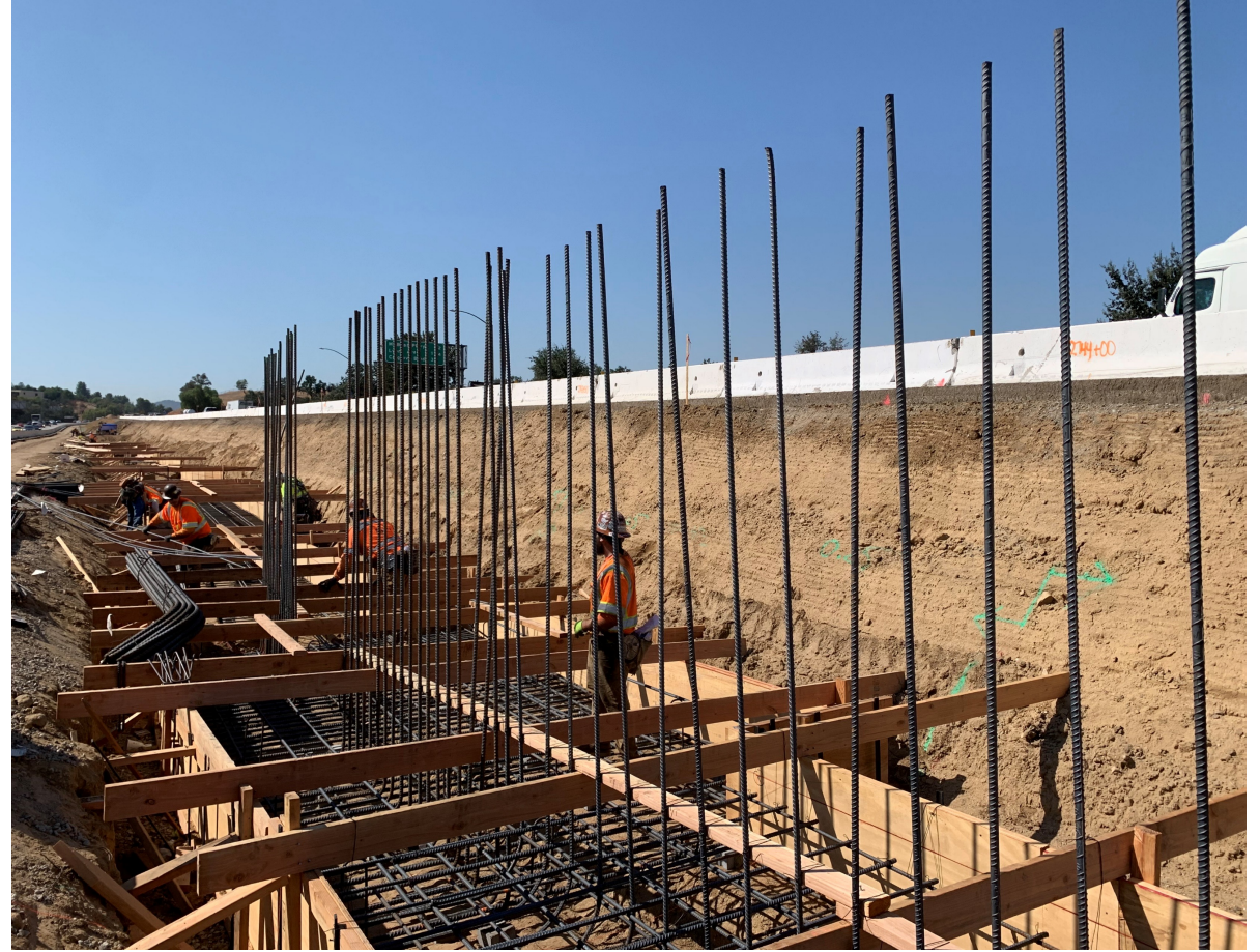
Footing and wall rebar activity in the I-5 center median at Valencia Bl
