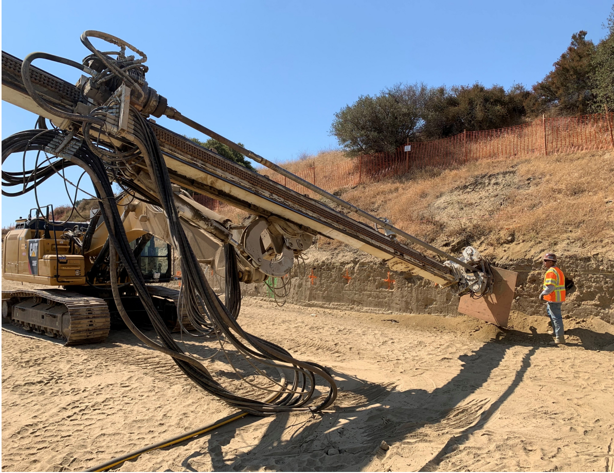
Soil stabilization (soil nail installation) in preparation for retaining wall construction along SB I-5
