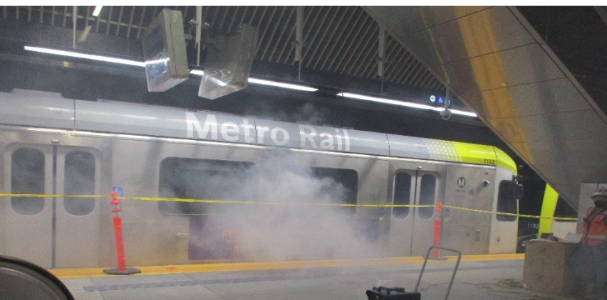
EXPO Station– Emergency Ventilation SIT
