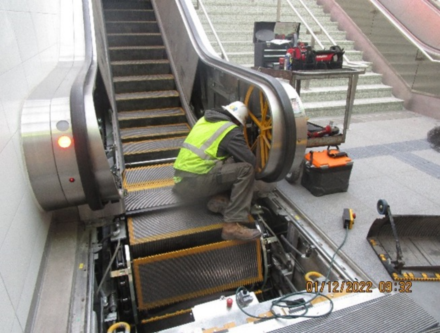
Performing final adjustments of speed controls for escalators in advance of final inspections
