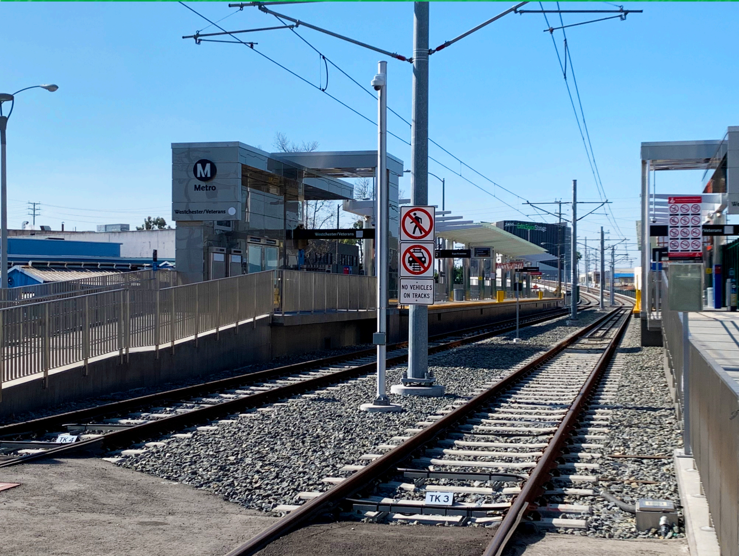
TVM canopy, Overhead Catenary System (OCS), railway track, and signage
