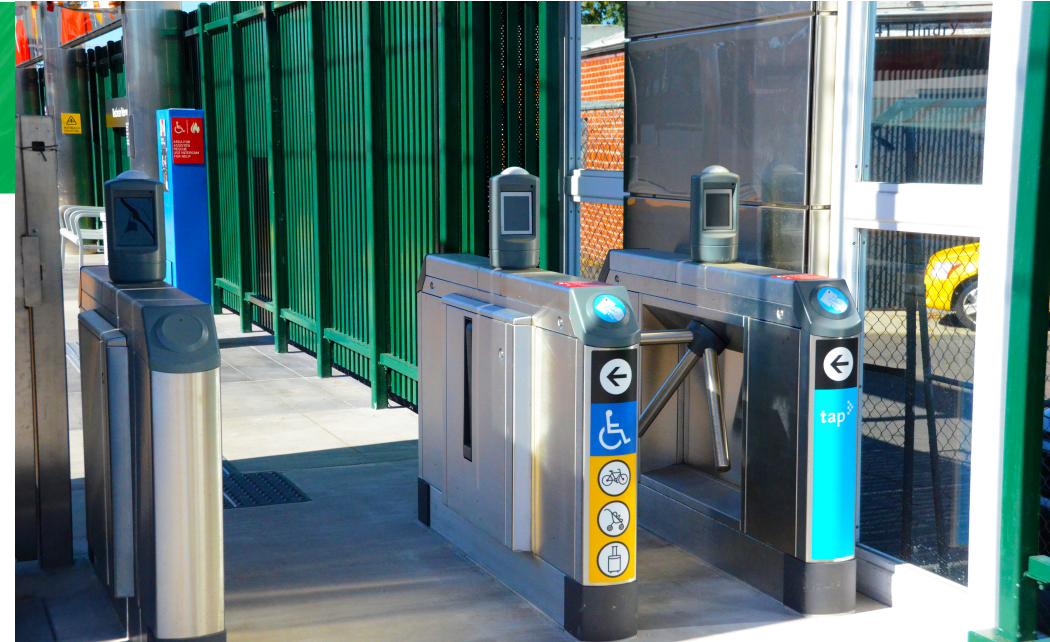
Installed fare gates at platform entrance
