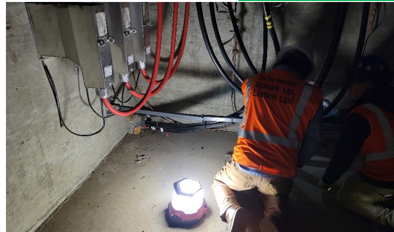
Remaining items Remedial work for TPSS #2 Vault
