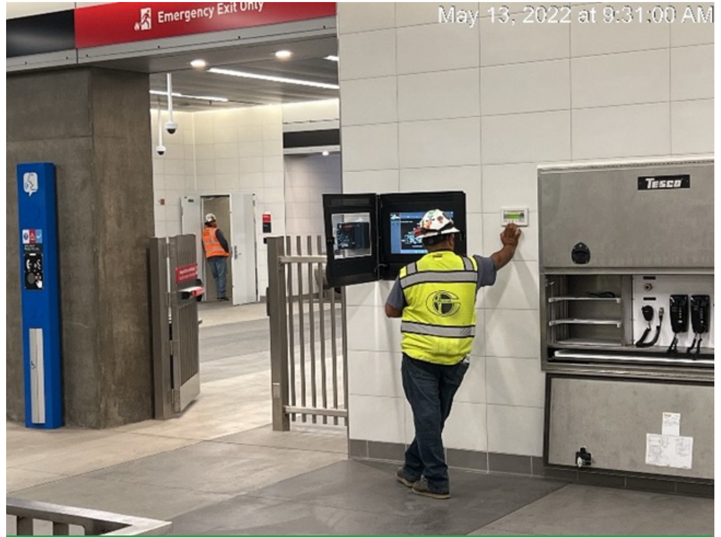
Fire life safety testing for smoke alarms at Leimert Park Station
