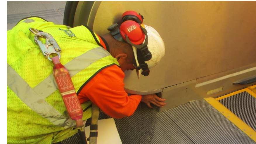
Leimert Park Station – Escalator SIT
