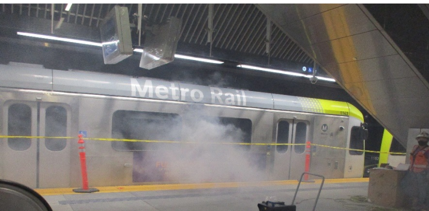
EXPO Station – Emergency Ventilation SIT
