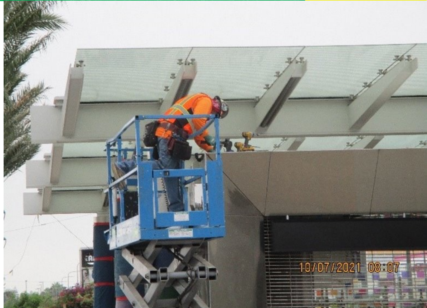
Installation of roof flashing above the main entrance portal at the station plaza
