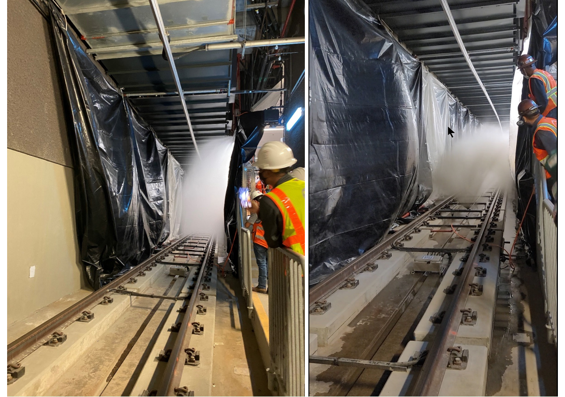
Over-Car and Under-Car Deluge System at Leimert Park Station
