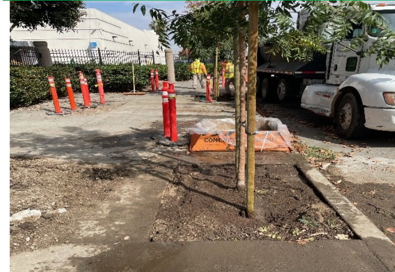
Unloading and planting trees along southbound Crenshaw Bl between MLK Bl/39th St
