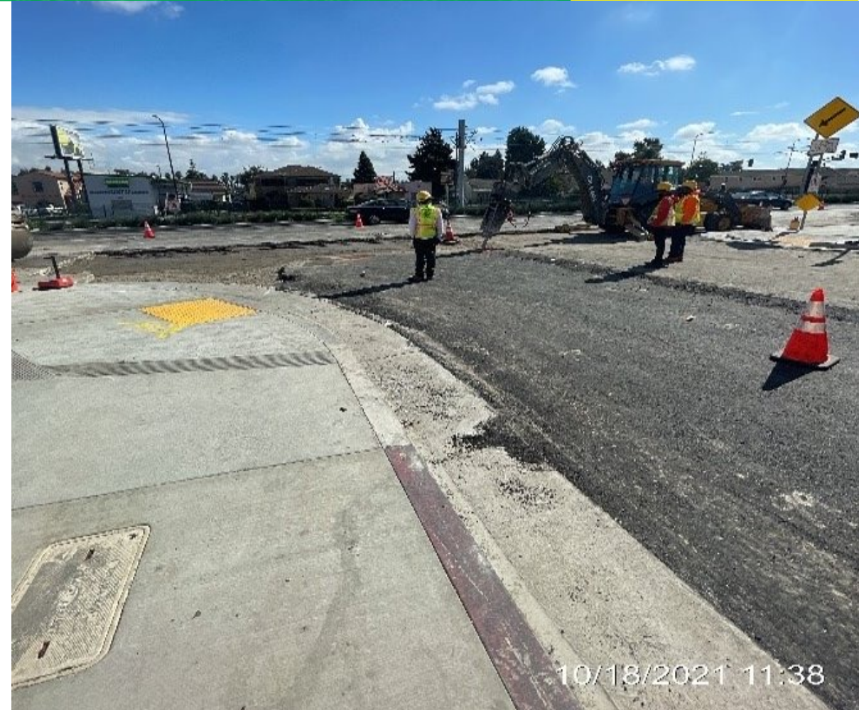
City of LA crews performing road restoration on Crenshaw Bl and Westmount Av
