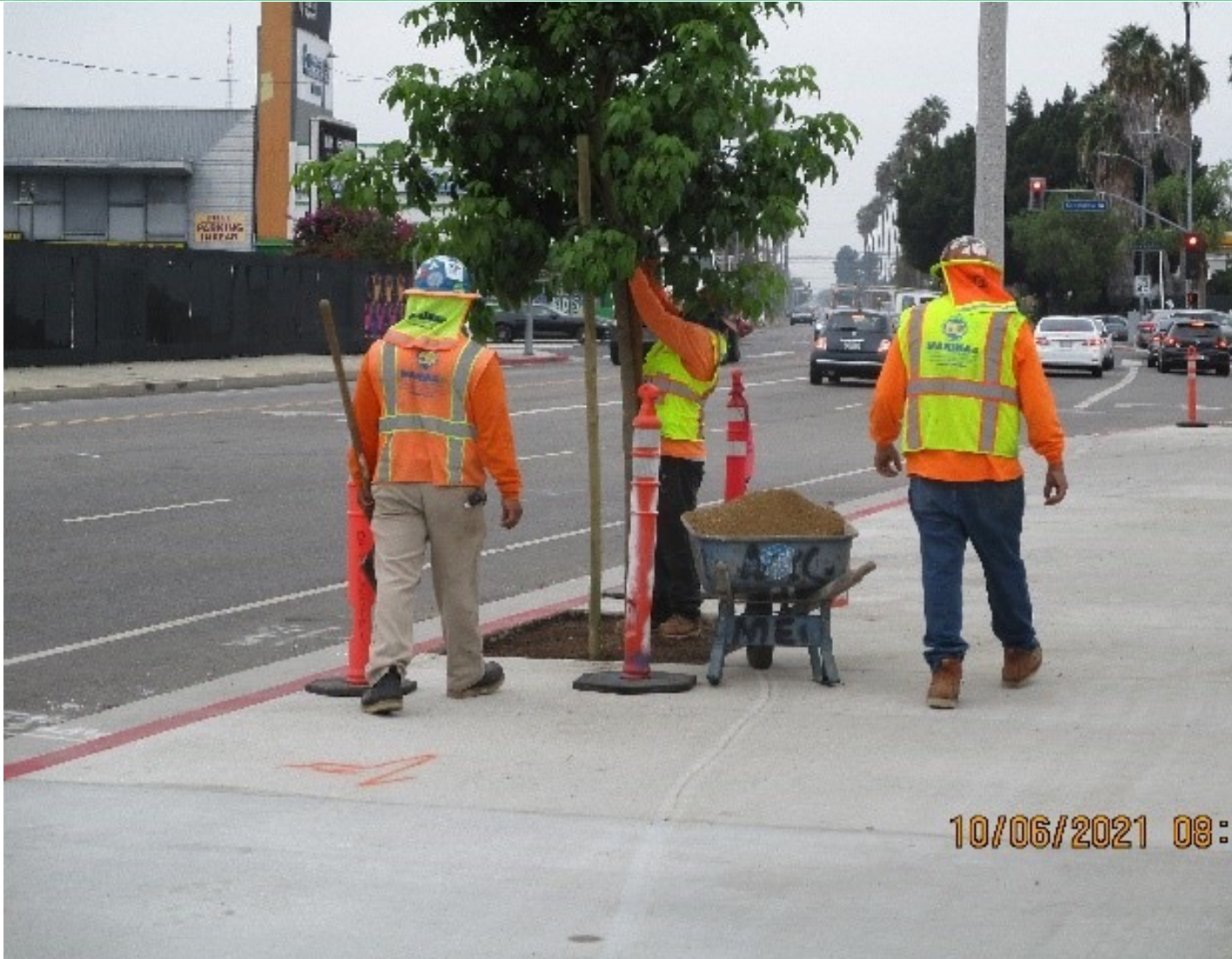
Spreading topsoil around the trees along westbound Obama Bl at Crenshaw Bl
