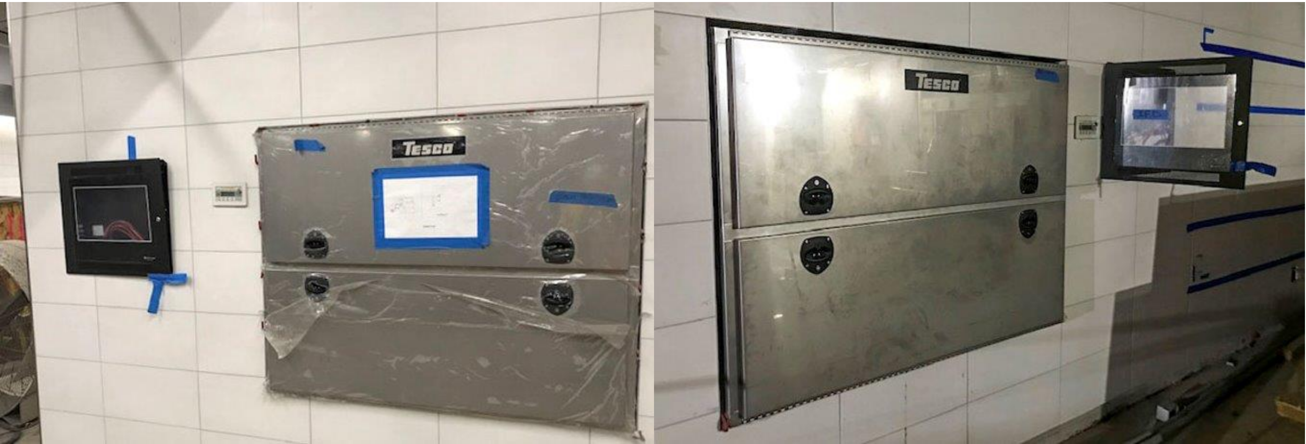
Emergency Management Panels (EMP)
