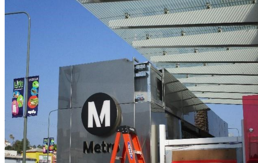
Stainless steel cladding panel installation at the main entrance plaza roll-up door
