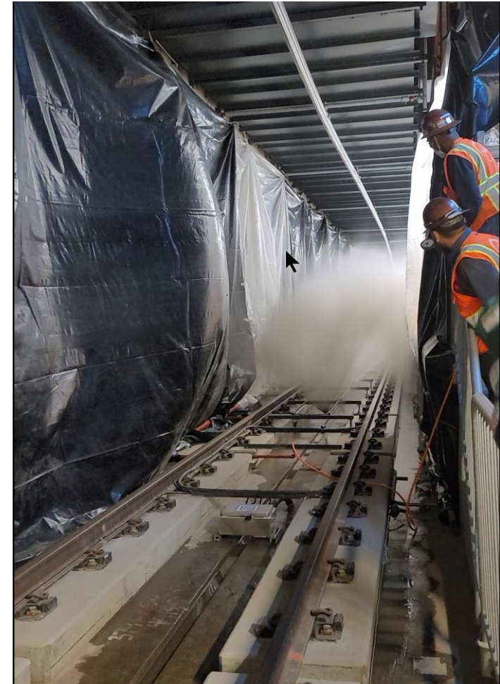
Under-Car Deluge System at Leimert Park Station
