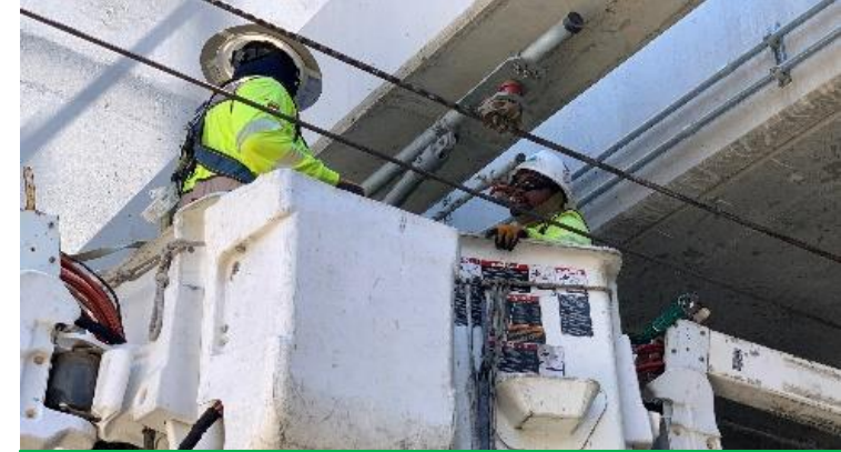
Remaining items walk for Over-Head Catenary System
