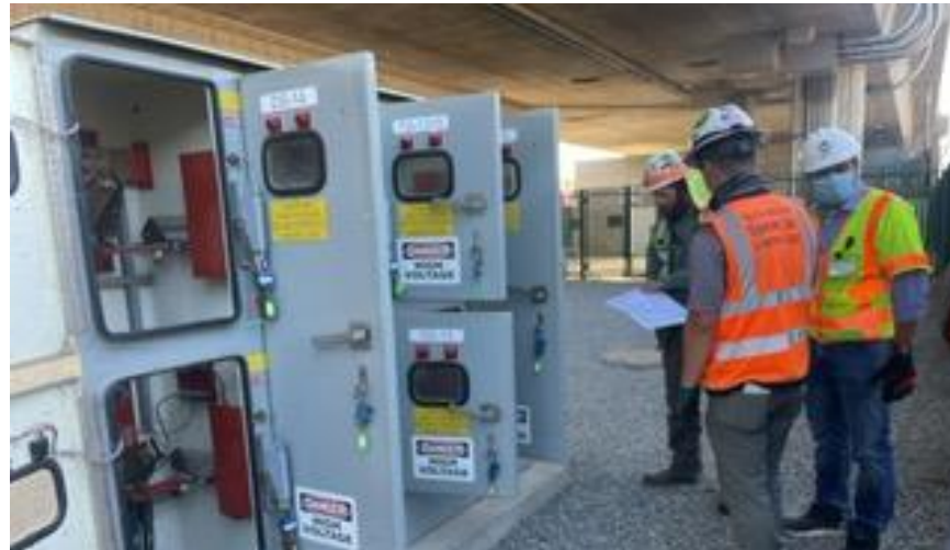
Remaining items walk for Traction Power Substations
