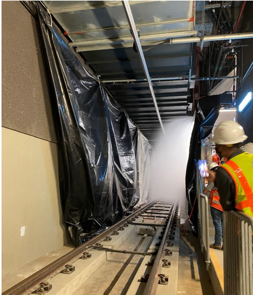
Over-Car Deluge System at Leimert Park Station
