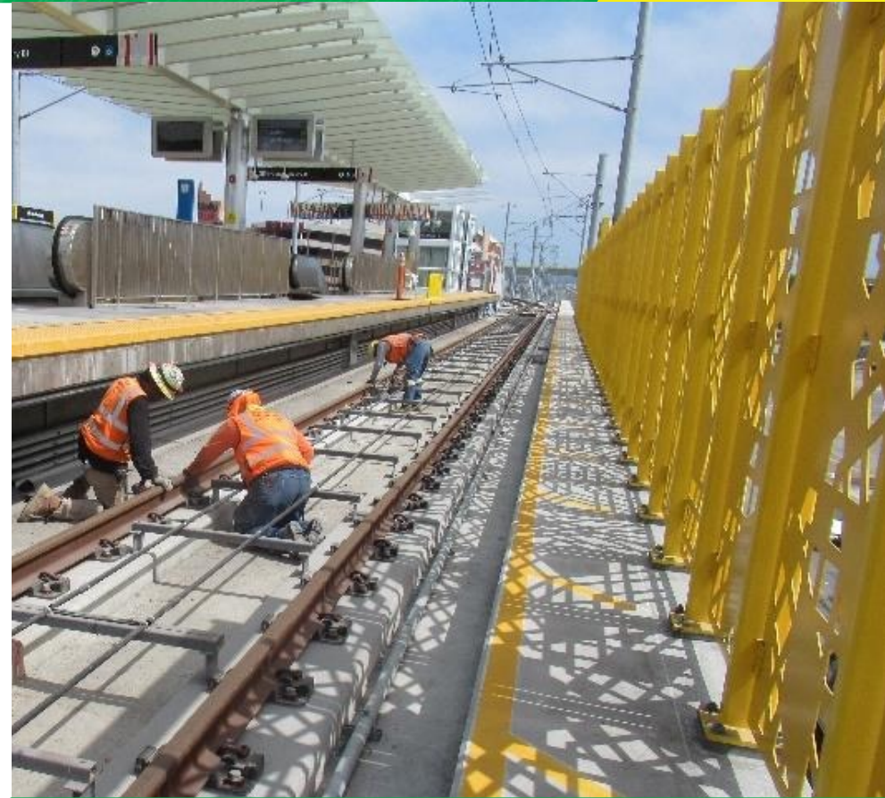
Workers preparing & applying new surface to NB track plinths on Century/Aviation bridge.
