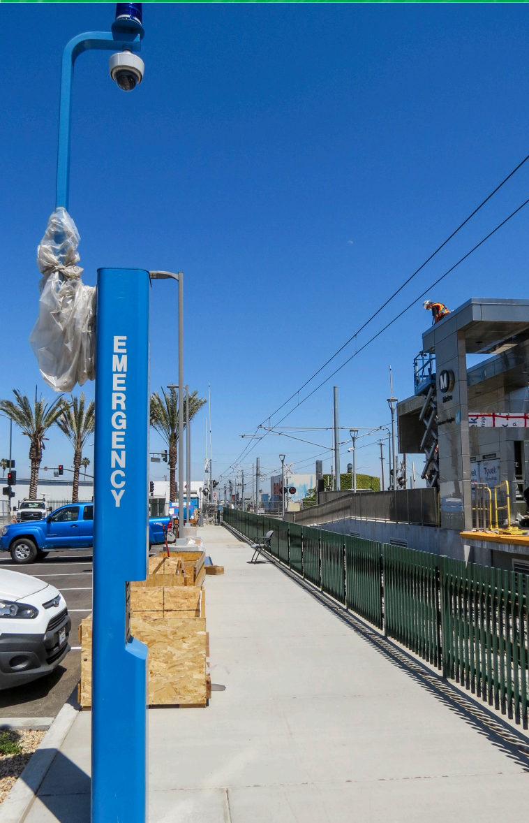
Emergency telephone (ETEL) with blue light station
