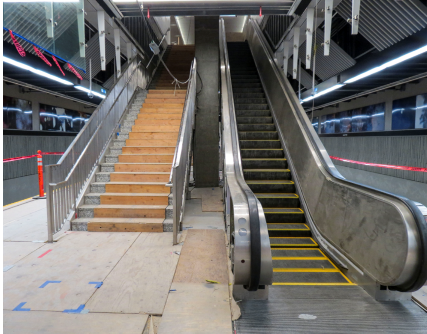
Leimert Park Station underground platform level with escalators, stairs, and artwork
