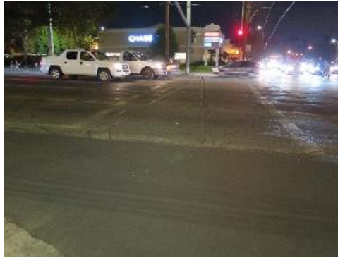
Figure 9: Faded and missing crosswalk striping at the intersection of Sepulveda Boulevard and Victory Boulevard.
