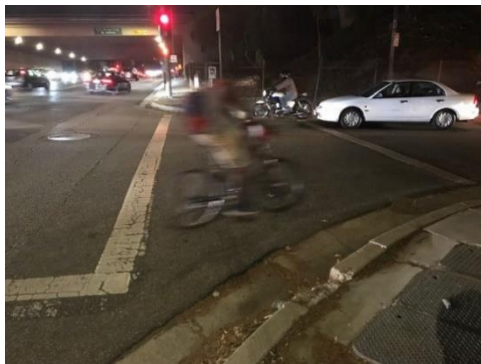
Figure 7: Broken curb ramp and faded crosswalk at Whitman Avenue and Victory Boulevard.
