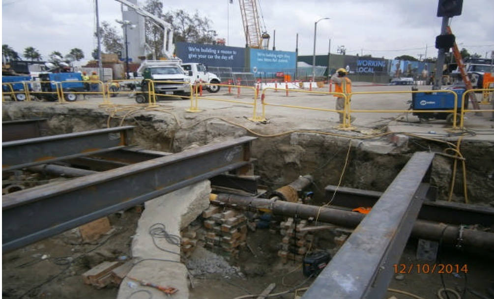
Steel Sleeve on Gas Main.
