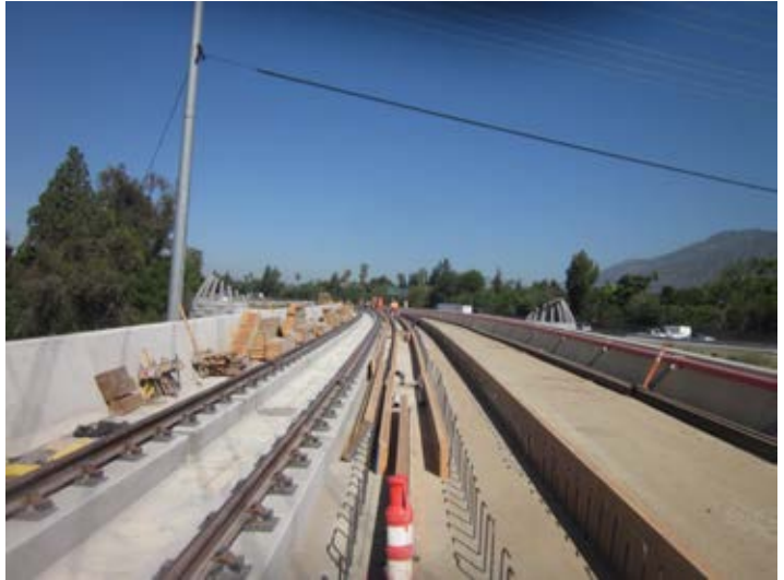
Segment 1: IFS Emergency Walkway and Ductbank
