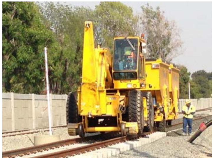
Segment 3: East of Buena Vista - Flooding Ballast
