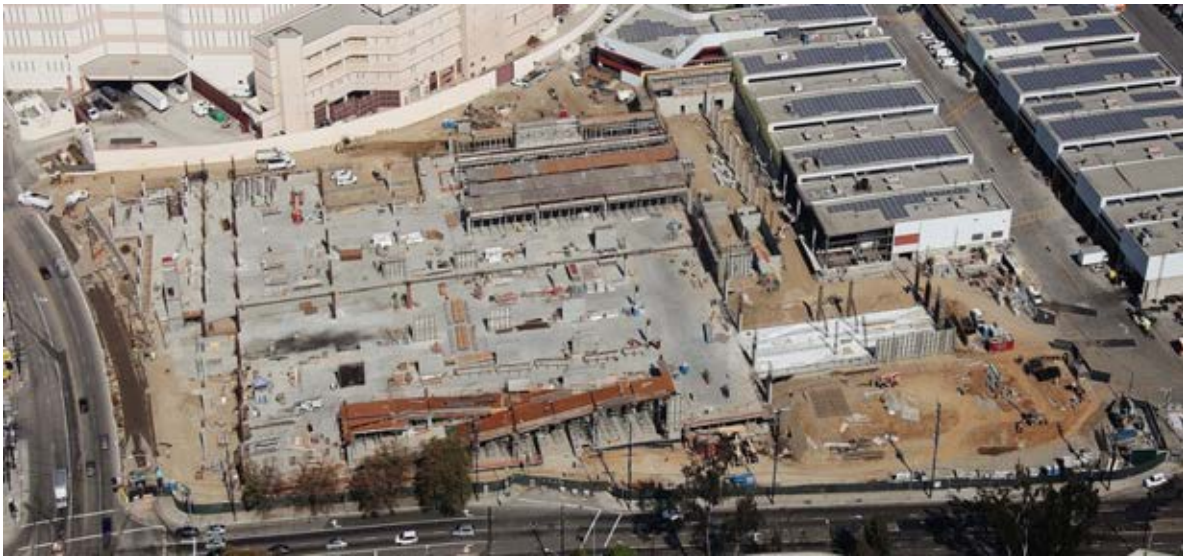
February 2014 Transportation Building, Parking Garage and Maintenance Building in construction; at the bottom side Cesar Chavez Avenue and at the left side Vignes Street.
