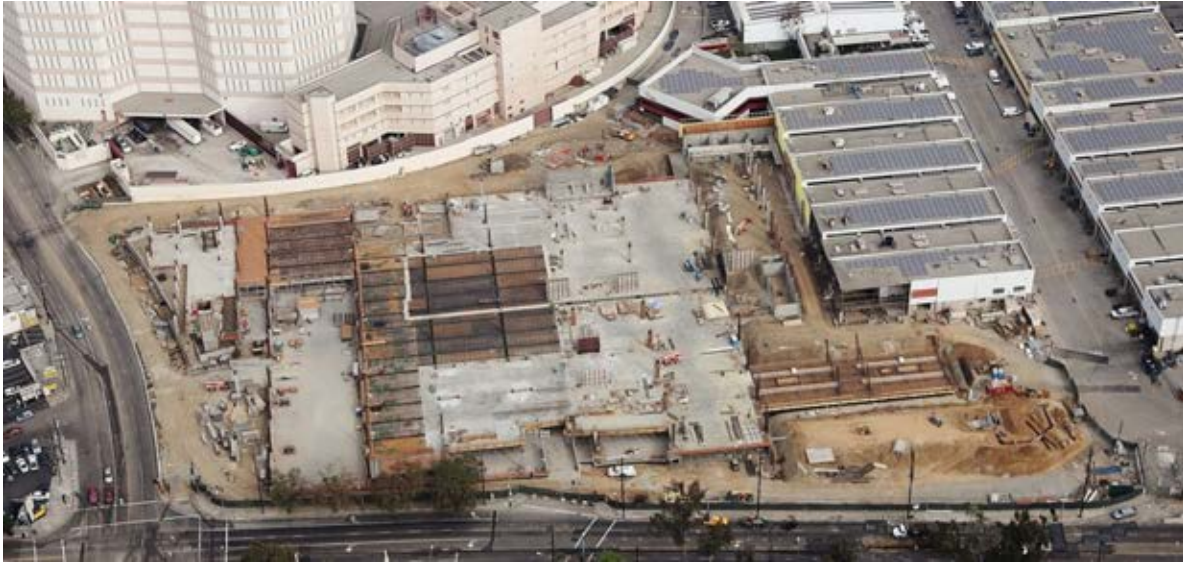
January 2014 Transportation Building, Parking Garage and Maintenance Building in construction; at the bottom side Cesar Chavez Avenue and at the left side Vignes Street.
