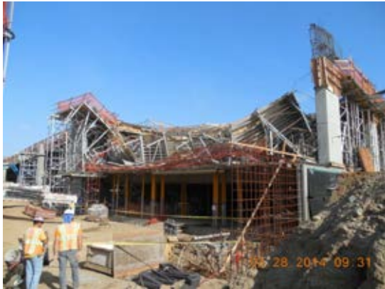
Roof Deck Pour No. 14 collapse Building B Roof Level.
