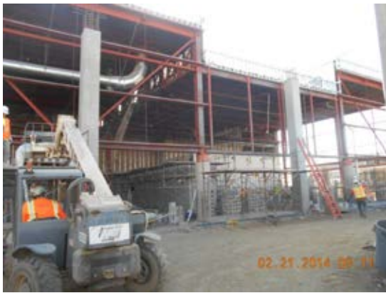
Placement of 1 st lift of exterior CMU walls at Old Radiator Shop.
