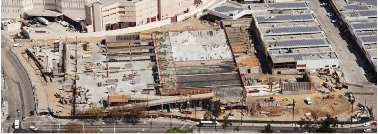
March 2014 Transportation Building, Parking Garage and Maintenance Building in construction; at the bottom side Cesar Chavez Avenue and at the left side Vignes Street.
