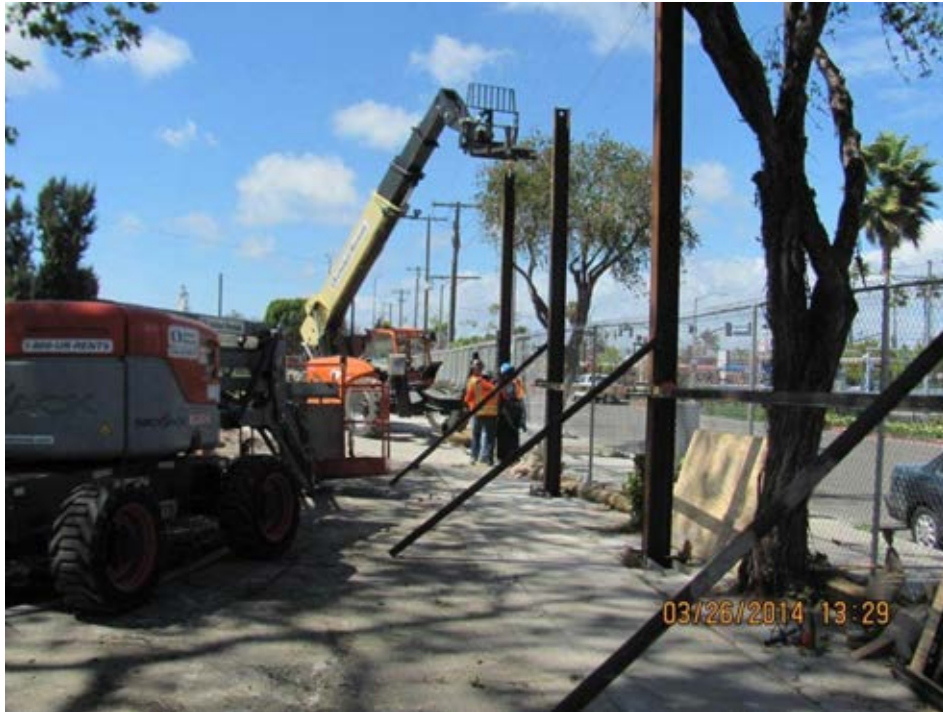
WSSC installation of I-beams for noise wall installation at Expo Station site.
