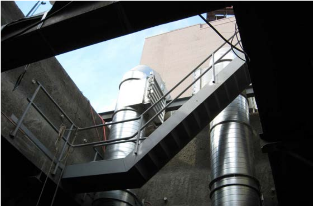
View of First Flight of Stairs to Landing on East Side of Exploratory Shaft
